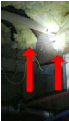
missing / displaced insulation
