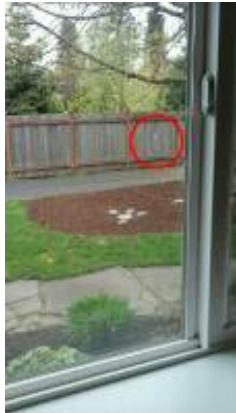
cracked / chipped window
