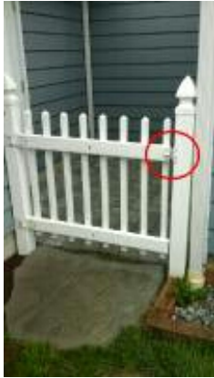
gate latch difficult to operate
