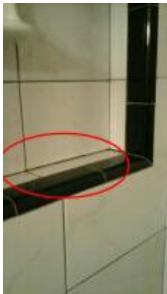
Recommend recaulking / regrouting shower
