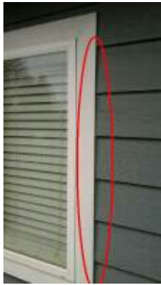
Repair/ replace caulking as needed.
