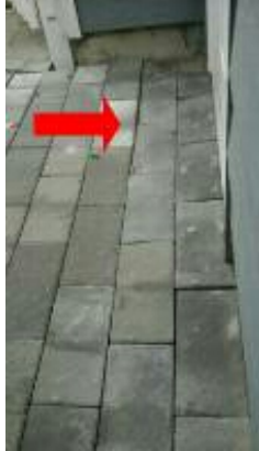
patio settling, trip hazard
