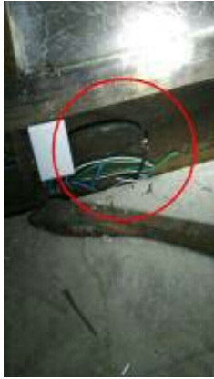
exposed wires, recommend repair
