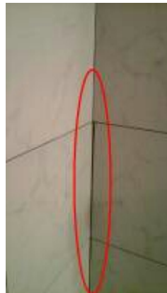
Recommend recaulking / regrouting shower
