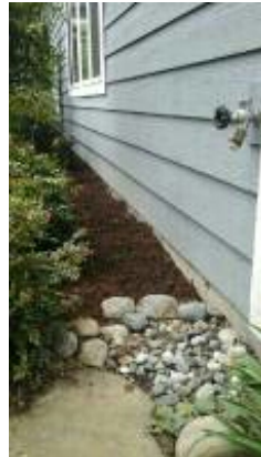
Recommend 4"-6" of clearance between siding & soil
