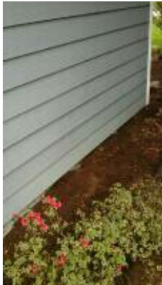
Recommend 4"-6" of clearance between siding & soil
