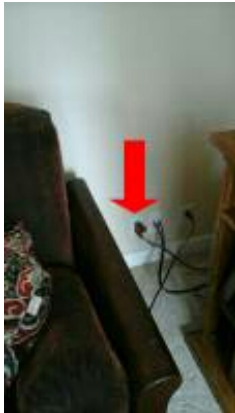
Outlet not operable
